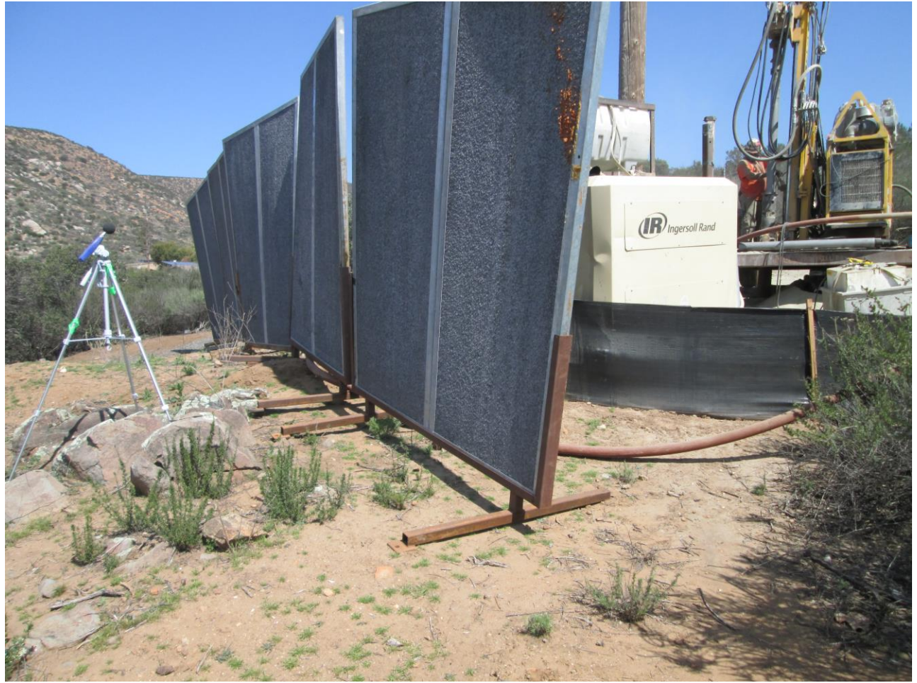
Photo 8: Noise Monitoring Equipment and sound walls were observed in place adjacent to micro pile drilling activities to ensure that noise levels during construction activities did not exceed thresholds at the nearest property line or adjacent to noise sensitive areas in accordance with MM NOI-2.
