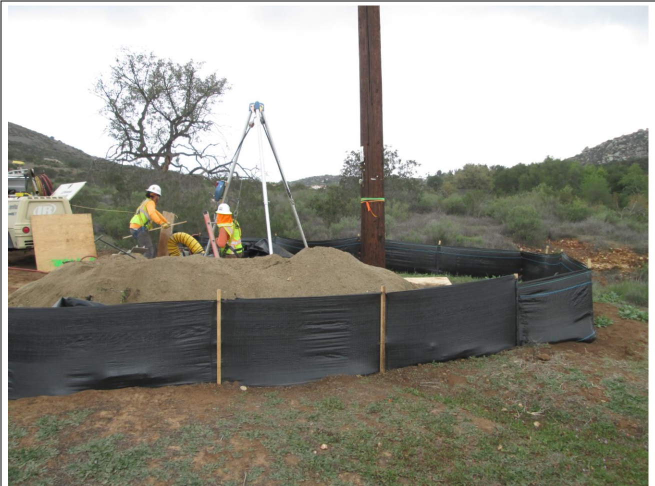
Photo 5: Crews were observed hand-digging pole sites within installed silt fencing required by the SWPPP.
