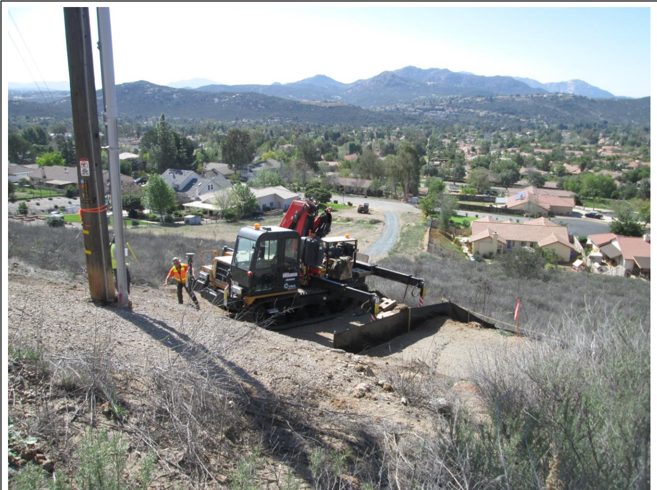
Photo 2: Crews were observed setting up equipment for micro pile foundation installation. Silt fencing was observed in the work area in accordance with the project SWPPP.
