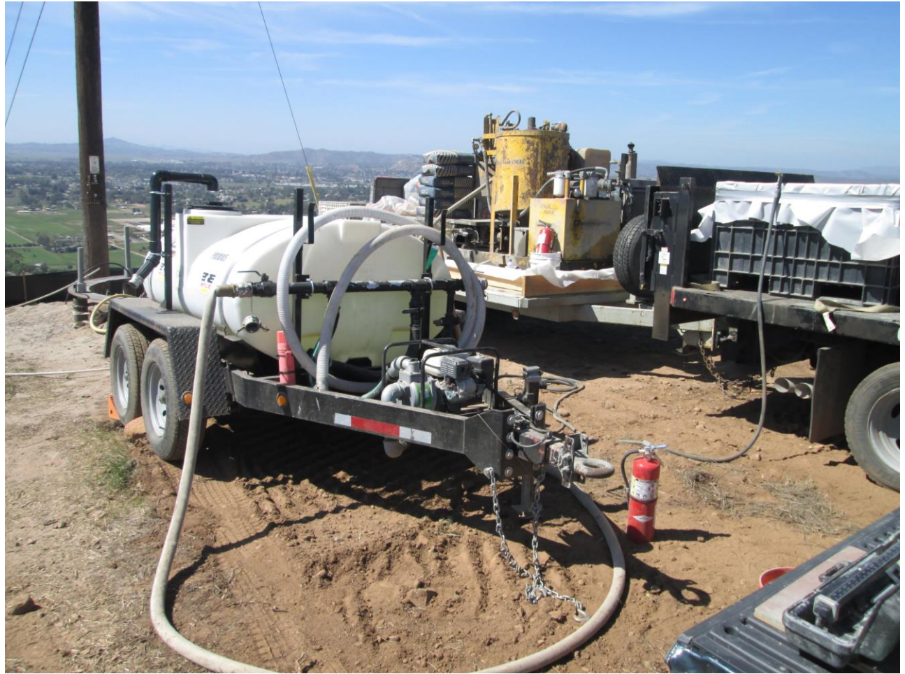
Photo 3: Crews were observed staging grouting equipment for micro pile foundations within approved work areas.
