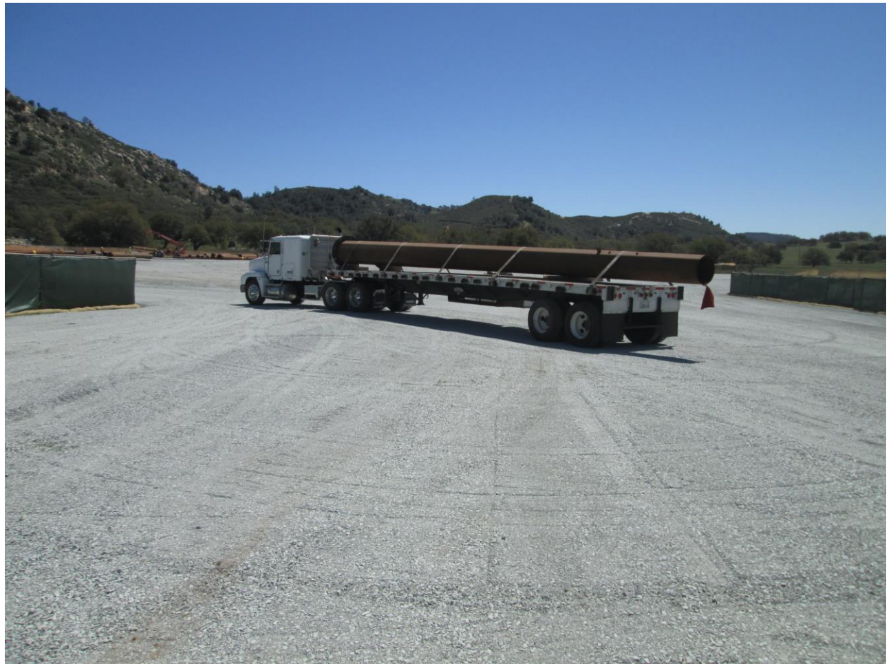
Photo 1: Staging Yards have been established and visual mitigation (opaque green mesh) and SWPPP mitigation (straw wattles, rock aprons, and gravel base) were observed installed. Deliveries for pole installation were observed at the staging yards.
