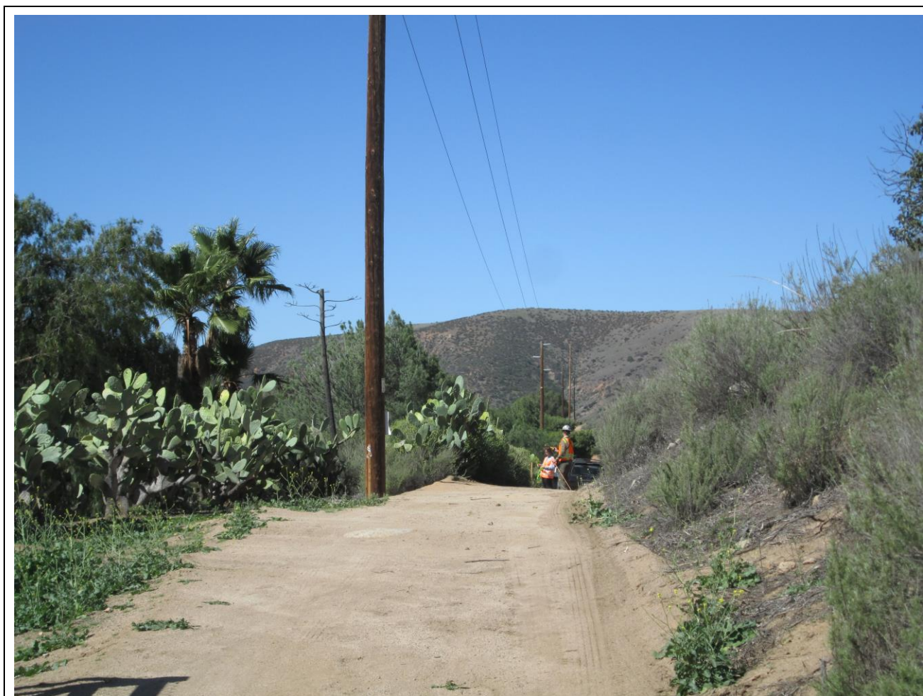
Photo 6: CPUC-approved biological monitors were observed conducting nesting bird surveys in accordance MM BIO-4 and conducting additional clearance sweeps prior to initiating ground work at pole locations.
